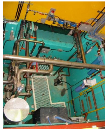
Fig. 4. Pump 's well.
